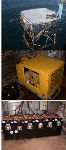
Power at COVE-CLH is self sufficient (off the grid). Some details (top to bottom) – solar panels (~4.5 Kw of solar panels) around COVE-CLH, a 7.5Kw diesel generator, and a bank of six 900 amp hour, 12 volt batteries wired in parallel.
